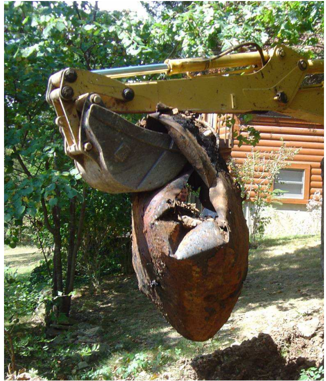
This deteriorated tank was still being used by the owners!
